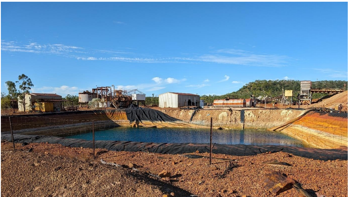
Image: Degraded infrastructure at Sandy Flat
