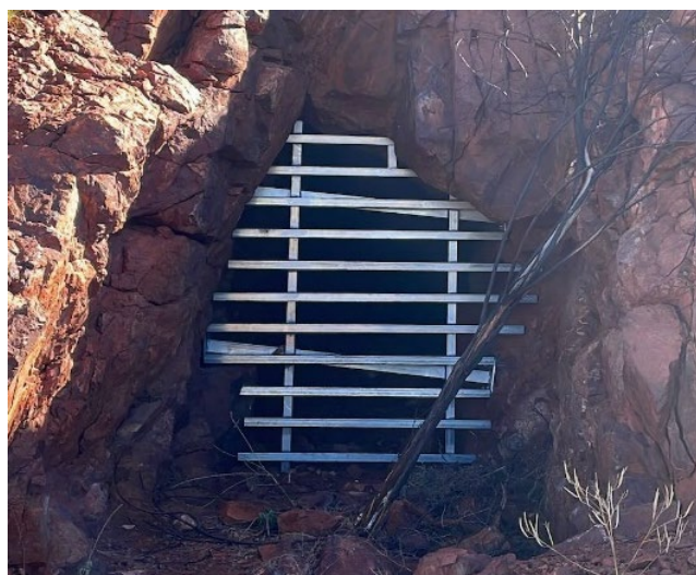
Adit covers enabling wildlife access
