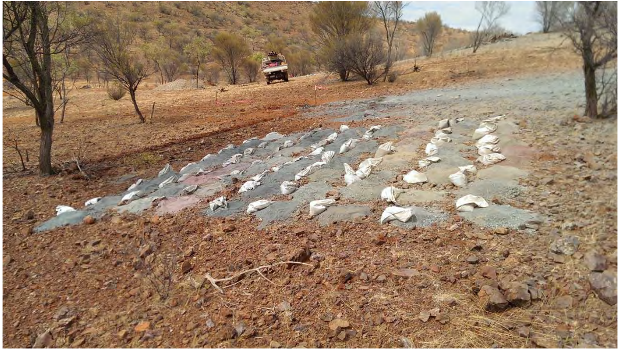
Figure 22. GGRC003 – rehab required
